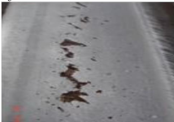
Figure 2: shows the image of the cracked rail to be used for the analysis
